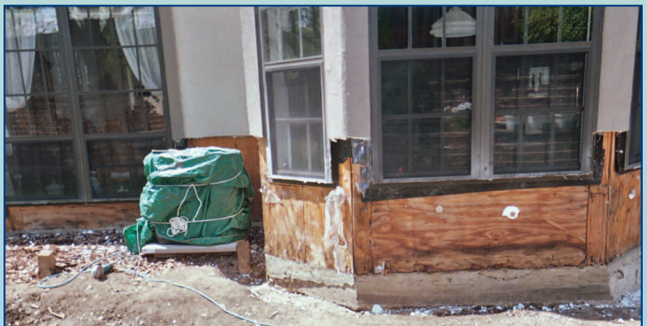
Example of damage that can occur to substrate when EIFS is improperly installed.
